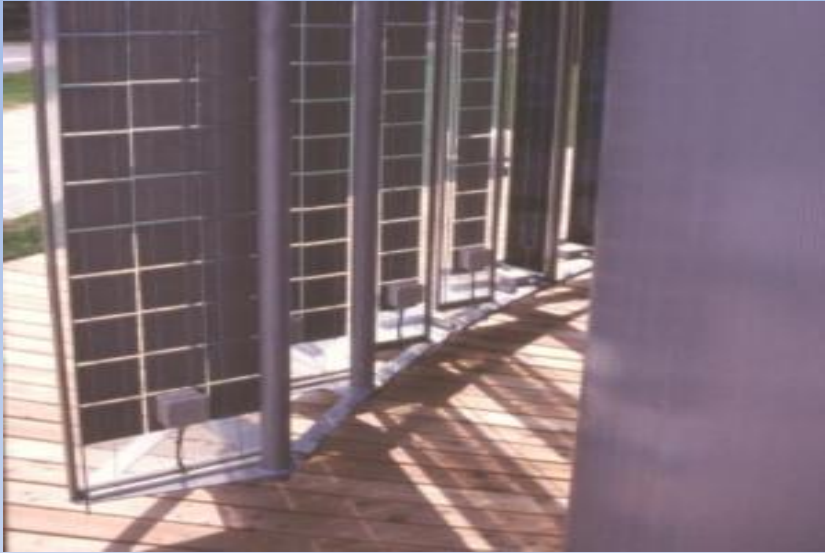
Vertical awnings with transparent solar cells in "Gemini Haus", Weiz, Austria (Photo: Denis Lenardic)
